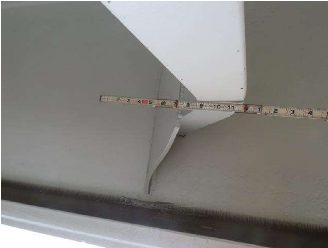
Span 2 Beam 1: Supplemental Inspection Impact Damage, Span 2 Bay 1, Diaphragm at Point of Impact Located 58 Foot From Bent 1 Has Crumpled. The Web of the Diaphragm is Distorted Up to 1 Foot. The Bay at the Point of Impact Around the Diaphragm has a Spacing of 75.5 Inches at the Top Flange and 67 Inches at the Bottom Flange. Only the Protective Coating Has Chipped and Cracked. (PAR)
