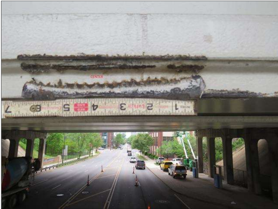
Span 2 Beam 1: Supplemental Inspection Impact Damage, The Bottom of the Beam is bent Northward for the Length of 35 Foot With the Max Distance at the Point of Impact Being 5.5 Inches. The Beam is Out of Plumb By 9 Degrees. The Point of Impact is 3 Foot 3 Inches Long and 2 Inches High and is Located in Span 2, 42 Foot 2 Inches From Bent 2. There are 3 Gouges at the Bottom of the Point of Impact: Left Gouge is 8 Inch X 2 Inch X 1/2 Inch, Center Gouge is 7 Inch X 2 Inch X 1/16 Inch, Right Gouge is 11 Inch X 2 Inch X 1/16 Inch. (PAR)
